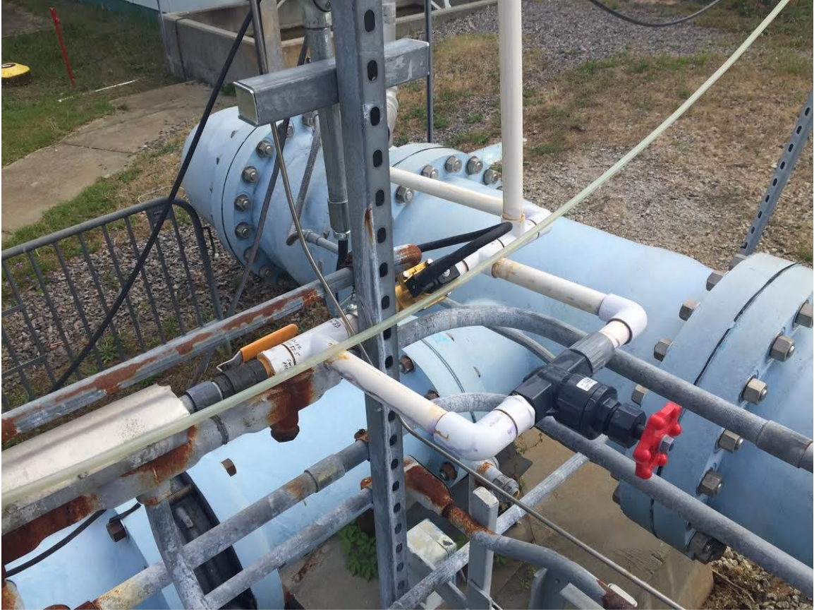
Figure A.5 New solenoid valve with bypass
