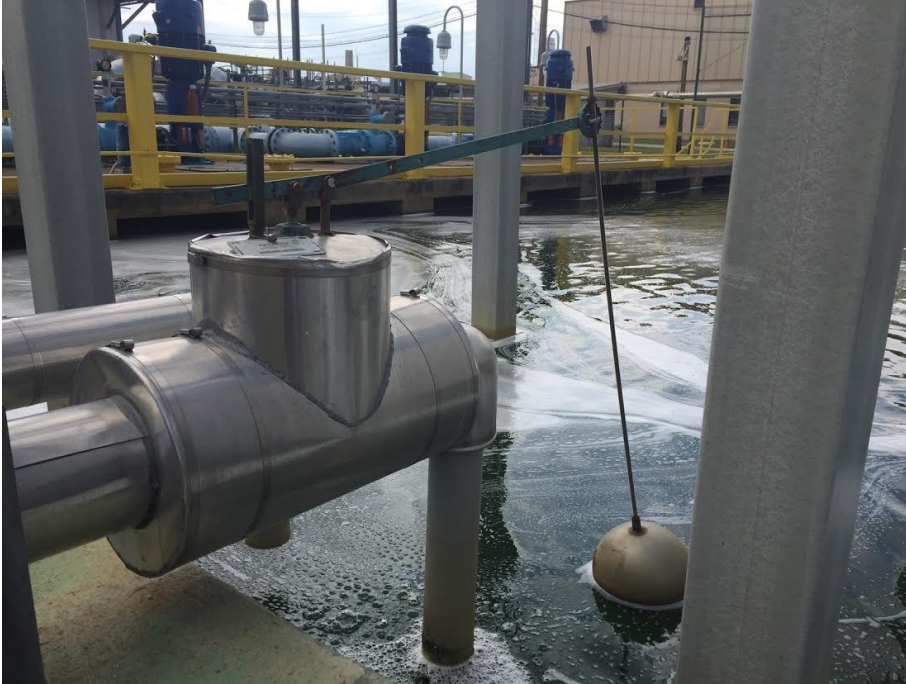
Figure A.3 Cooling towers Level Control Float
