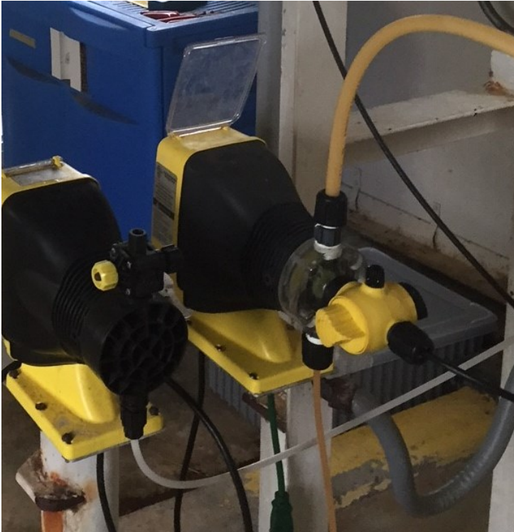
Figure 1.5. CL-49 Metering Pump
