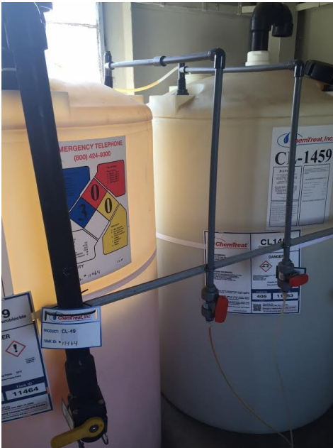
Figure A.2 Chemical Tanks; Left CL-49 & Right CL-1459 (not in use)
