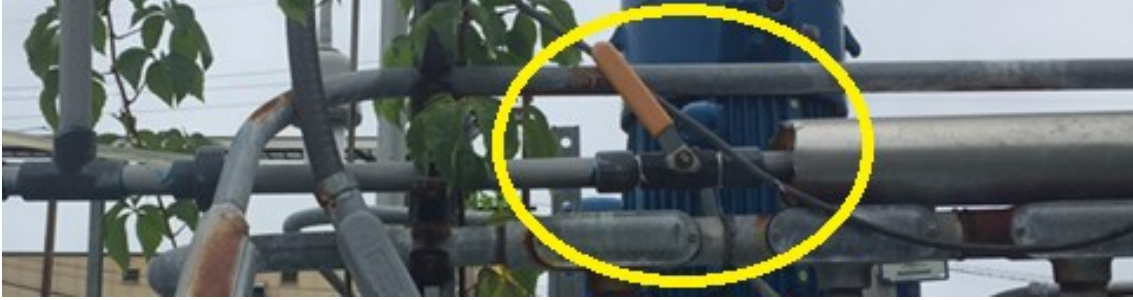
Figure 1.4. Blowdown valve throttled
