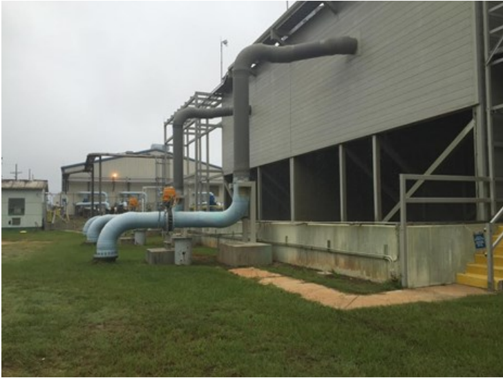
Figure A.1 Cooling towers
